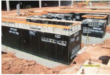
Figure 14 - Precast UPS pits
