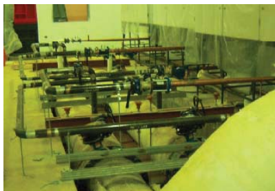
Figure 12 - Chilled water piping
